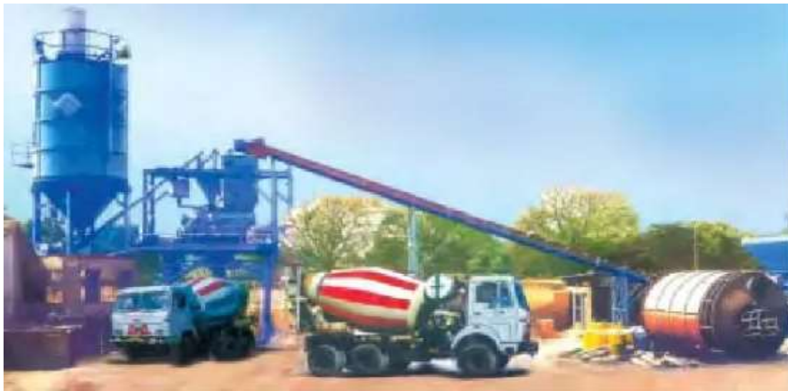
Modern ready mixed concrete plant.
