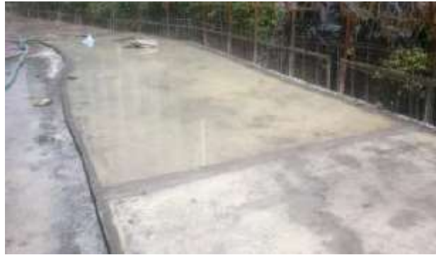
Fig:16 Ponding of slab
